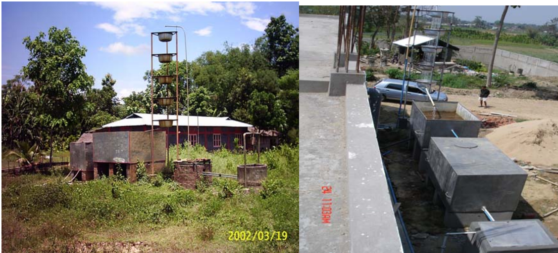
An old Iron removal plants installed in a village in Dimapur District
